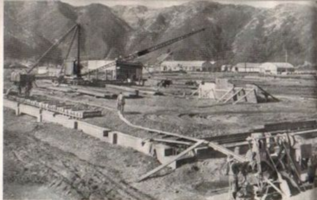
This photograph, taken on May 9th, 1936, shows the Factory foundations taking shape.
