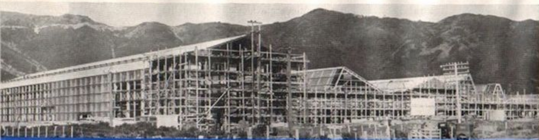
On the left is shown the huge structure nearing completion, as at 9th October, 1936.
