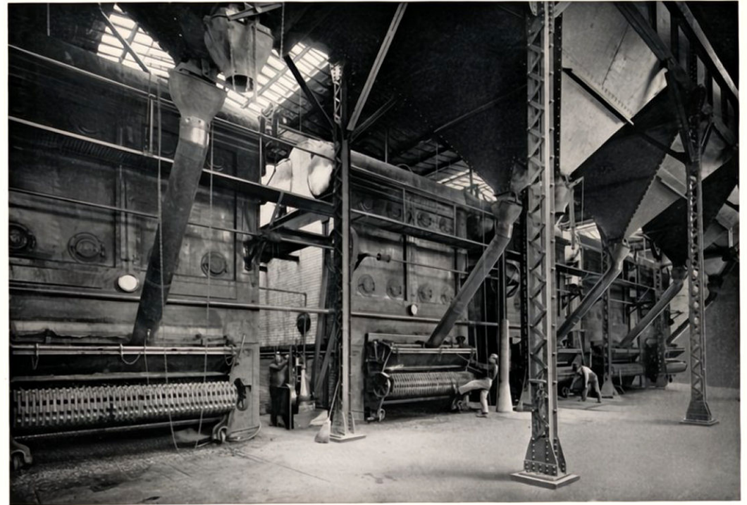
The big battery of boilers in connection with the Jeffery power plant, showing automatic coal carrying apparatus and stokers
